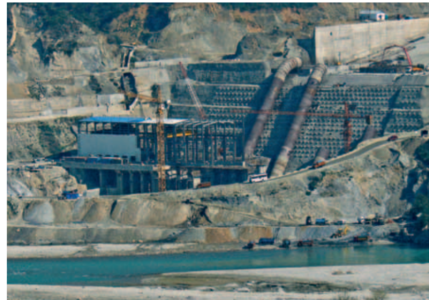
Tehri Dam project in Uttarkhand, India, led to a big public protest, but it was completed in 2006 and the reservoir submerged the homes of more than 100 000 people. There are several new projects on-going in the region. This photo is from a construction site of a dam on Alaknada river near Srinagar.
